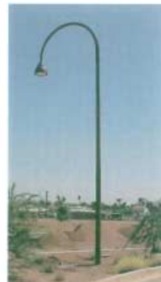
Photo 36. Overhead vehicular driveway light. Cast concrete shaft-metal arm.
